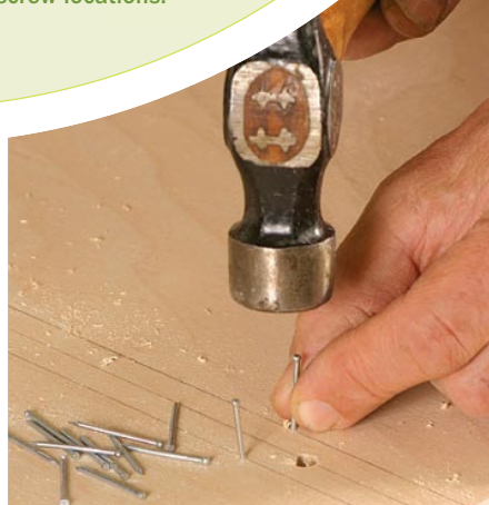
Brads are helping hands. Brads driven in along the edge lines will hold the intersecting panel in place as you transfer the location of the clearance holes. A pair at the top and at the bottom is all you need.
